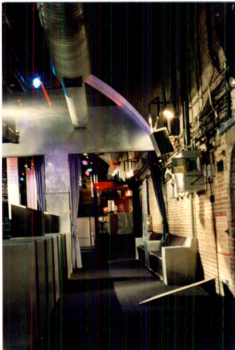
Fig. 16 Tunnel nightclub, uncovered wiring and pipes
